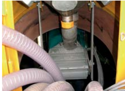
▲ Loading hopper, equipped with a dust extraction system
