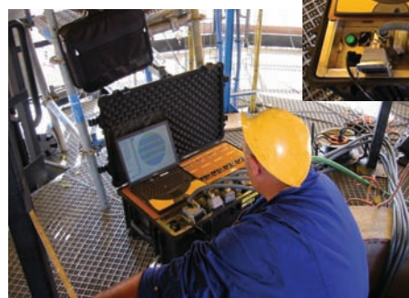
A Mourik employee monitors the progress of pressure drop measuring.
